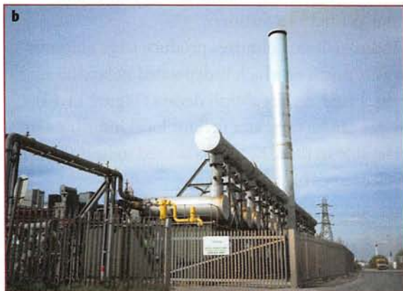
Figure 11.13 a Deep in the waste of landfill sites, methane gas accumulates and must be burnt off or it could become dangerous – a landfill flare-off. b Alternatively, a power-generating plant can be set up at a landfill site to generate power for the local area.
