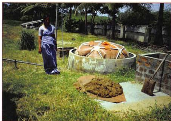
Figure 11.12 A small-scale biogas generator uses animal waste to produce methane for a village's needs.
