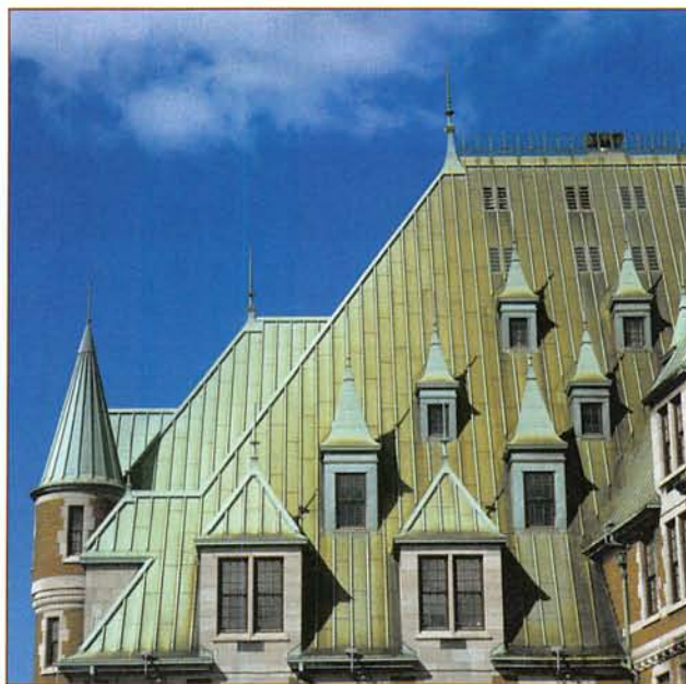
Figure 8.9 The copper sheets of this roof have become coated in a layer of green copper(II) carbonate.
