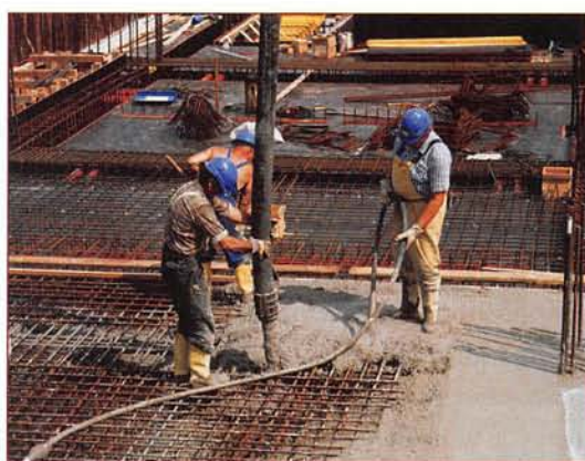
Figure 9.27 Construction workers using a pump to lay concrete around a mesh of metal rods. The rods will strengthen this reinforced concrete.
